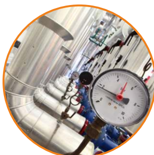
Heat exchange unit
