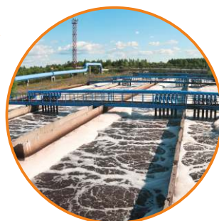
Sewage treatment plant
